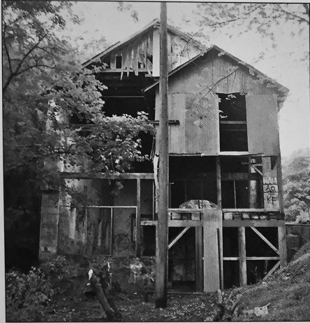
Much of the original downstream walls had been destroyed by the time restoration began in 2003.
